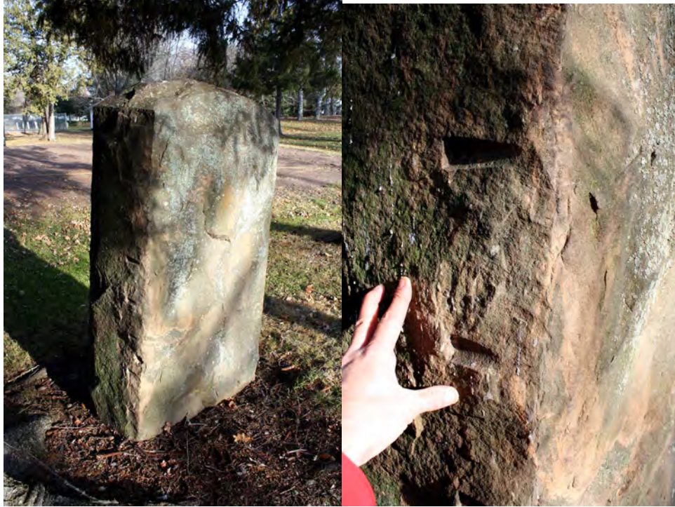
The Dr. P. N. Fenger monument in the Askov City Park is comprised of Hinckley Sandstone and having been erected in 1927 serves as an excellent weathering control sample. The drill holes present on the sides indicate a man-made surface.
